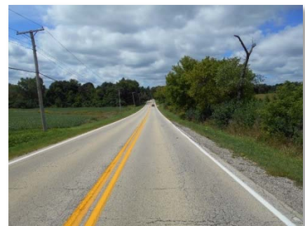
Minimal shoulders and typical pavement failure
