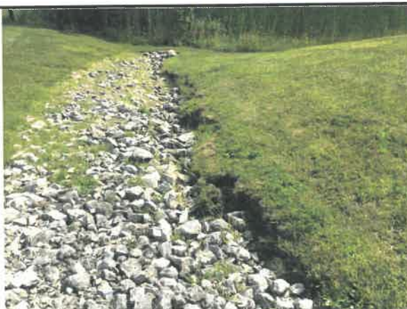
Side of trench eroding away
