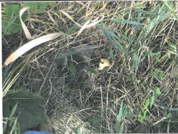
Outfall structure fully submerged in sediment
