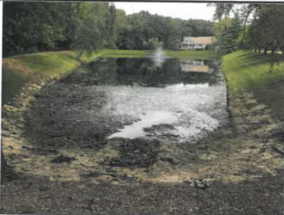
Accumulated sediment/ debris in storm inlet pipes on southerly side of basin
