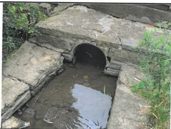
Outfall discharging into the basin. The outfall is in poor condition and sediment was observed in and outside of the outfall.
