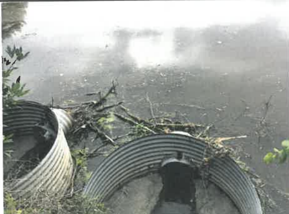
Accumulated debris at outfall structure
